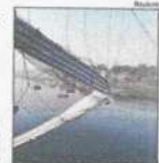
The suspension bridge in Morbi, Gujarat, collapsed on October 23, 2022, during heavy rain.
